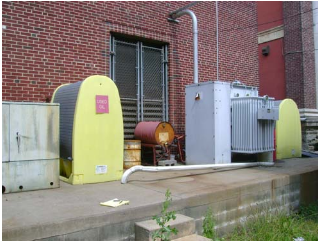
Transformer & Materials Mgmt.
