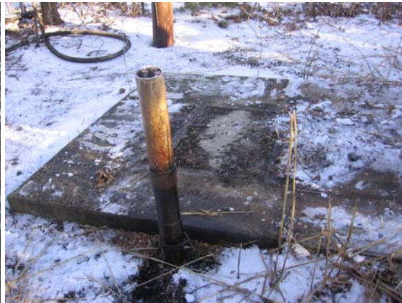
PCB Laden-Oil Leakage
